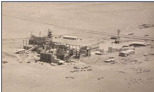
13 An Image Taken in 1956 Documenting the Construction of Al-Yamamah Cement Company's Factory.
